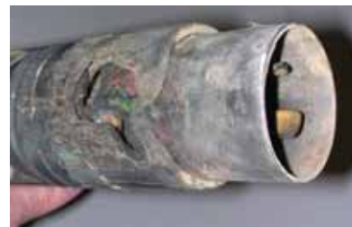
Non-watertight plug failure due to water getting into wiring chamber.
