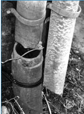
Steel U-Guard requires grounding strapping and does not have belled ends.
